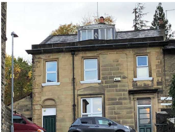
Image 2 - Unsightly and Difficult to Maintain Front Dormer
