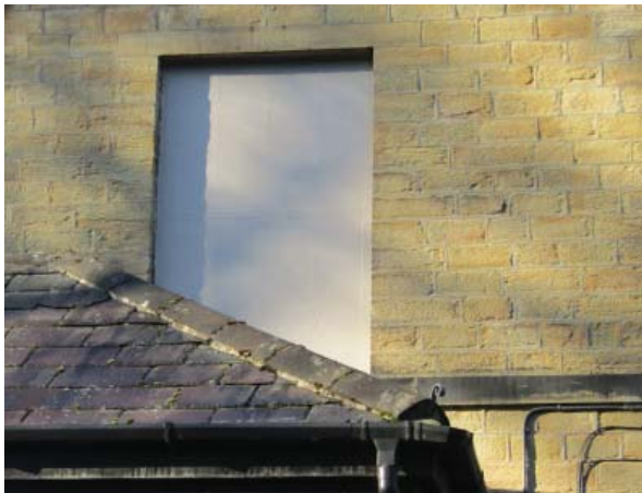
Example of blocked window above orangery.
