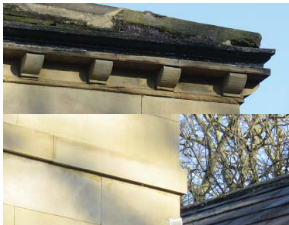
Modest decoration. (Above) the dental course and gutter. The hip showing damage. (Below) sill level detail.
