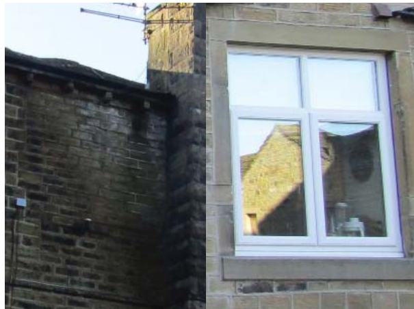
view of staining and odd coursing to rear elevation. Kitchen window display different treatment and detailing.
