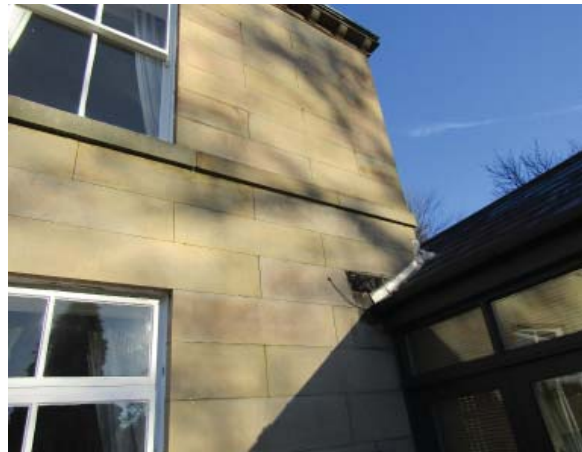
View of what could of been a flat roof next to the leading of the orangery roof at eaves height.
