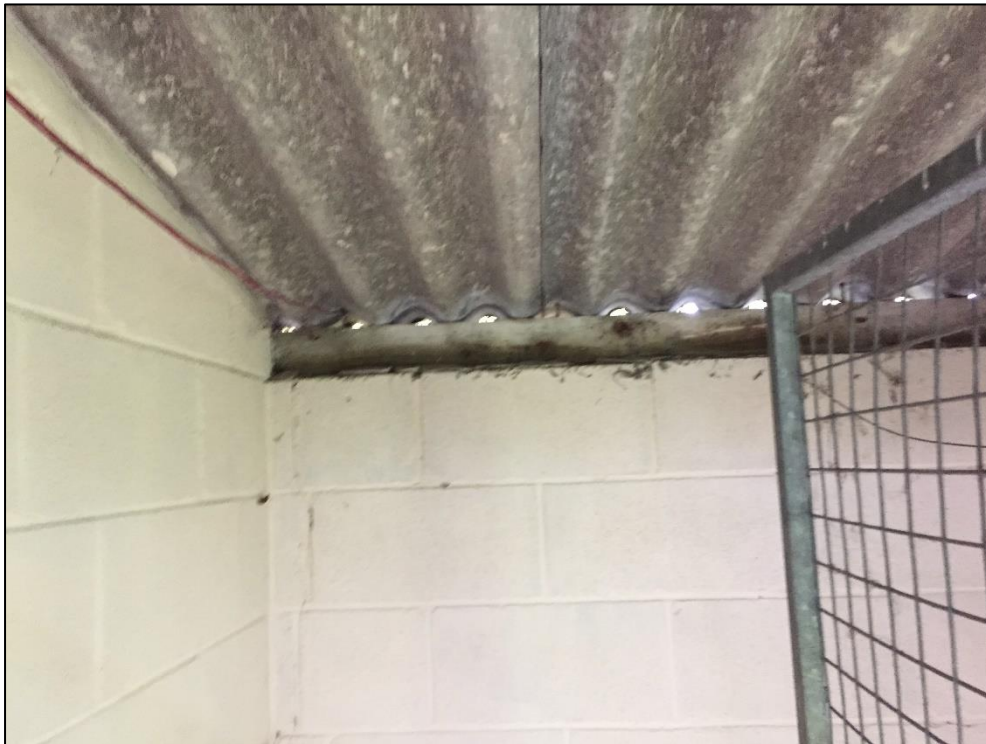
Plate 12: Interior gaps in the roof of the isolation kennel
