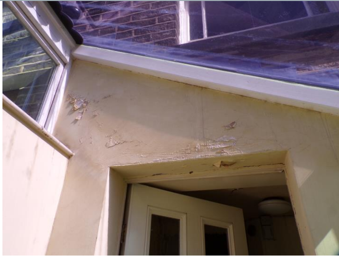
Evidence of damp to the conservatory
