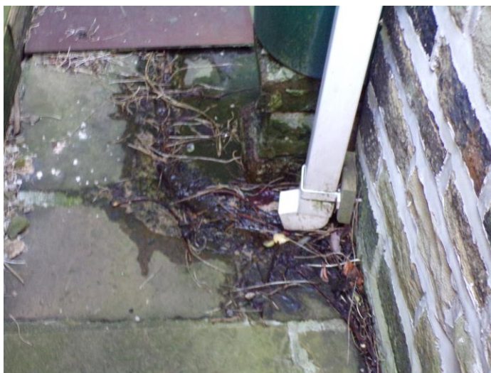
Blocked gulley / drain
