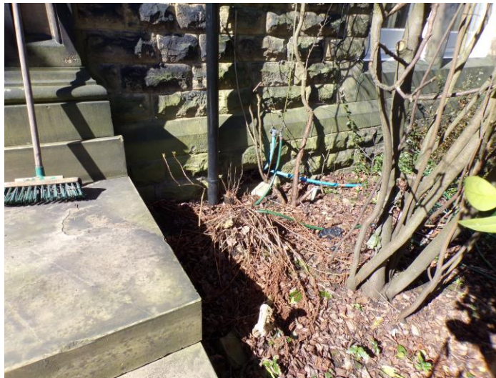
Ventilation to sub-floor
