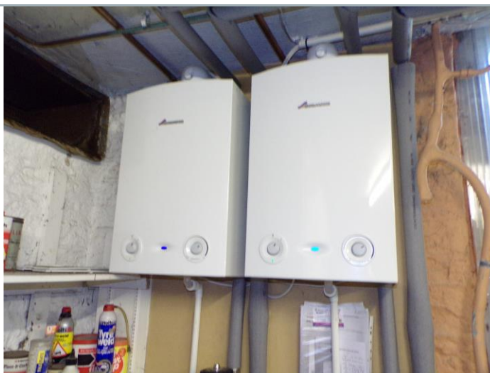
Dual boiler system
