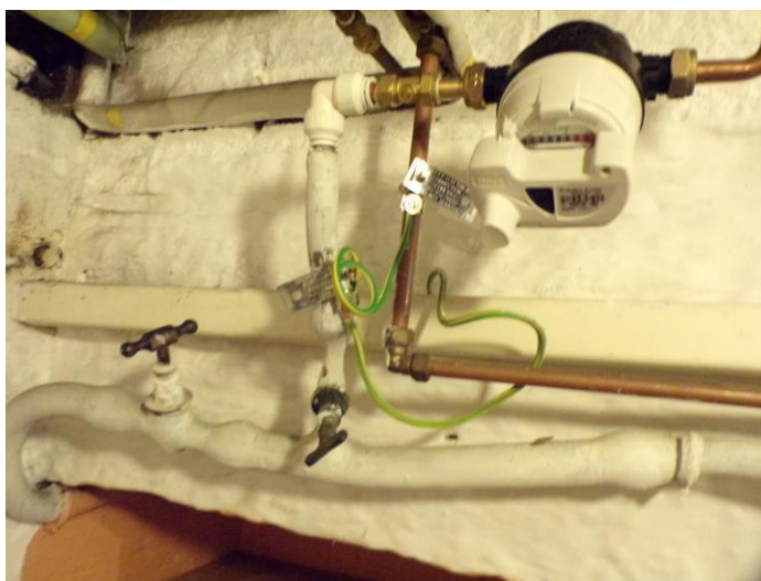
Water stop tap and meter
