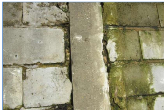
Photo 4 - Crevices within masonry of building 1 south elevation (damp walls).
