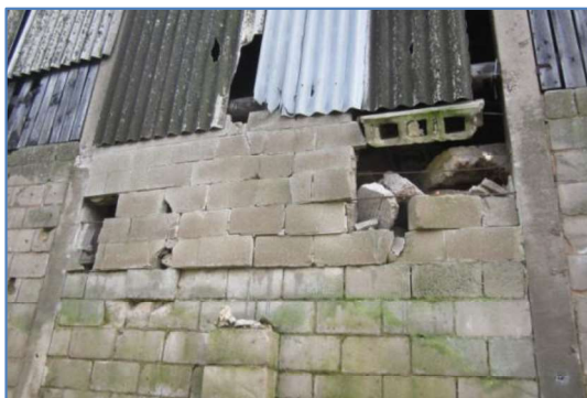
Photo 5 - Block work in poor condition on west elevation to building 1.
