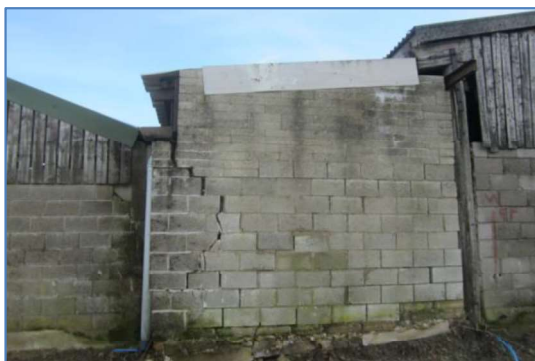
Photo 13 – West elevation of building 6, showing large cracks in rear wall.
