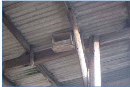
Photo 20 – Box attached to timbers in building 9.
