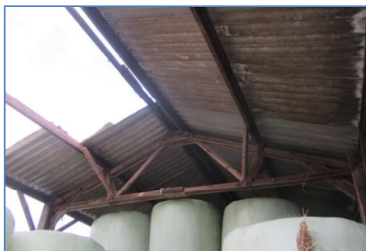
Photo 18 – Partly collapsed/missing roof of building 8, and thin roofing timbers.
