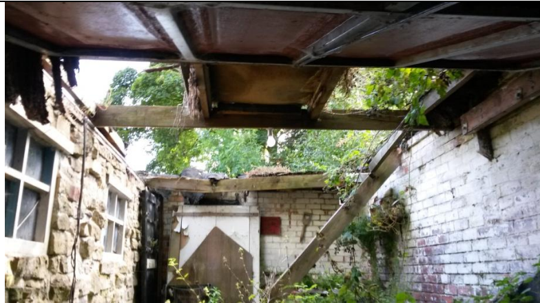
Photo 8: B4 internal view showing collapsed roof
