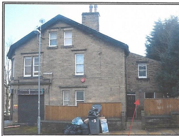
Structural Movement 1, Macauly Road, Birkby, Huddersfield.
