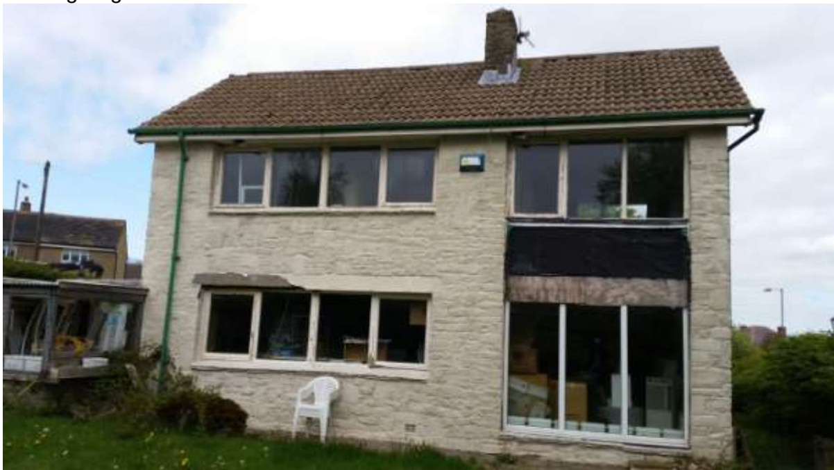
Rear view of existing host building showing signs of dilapidation
