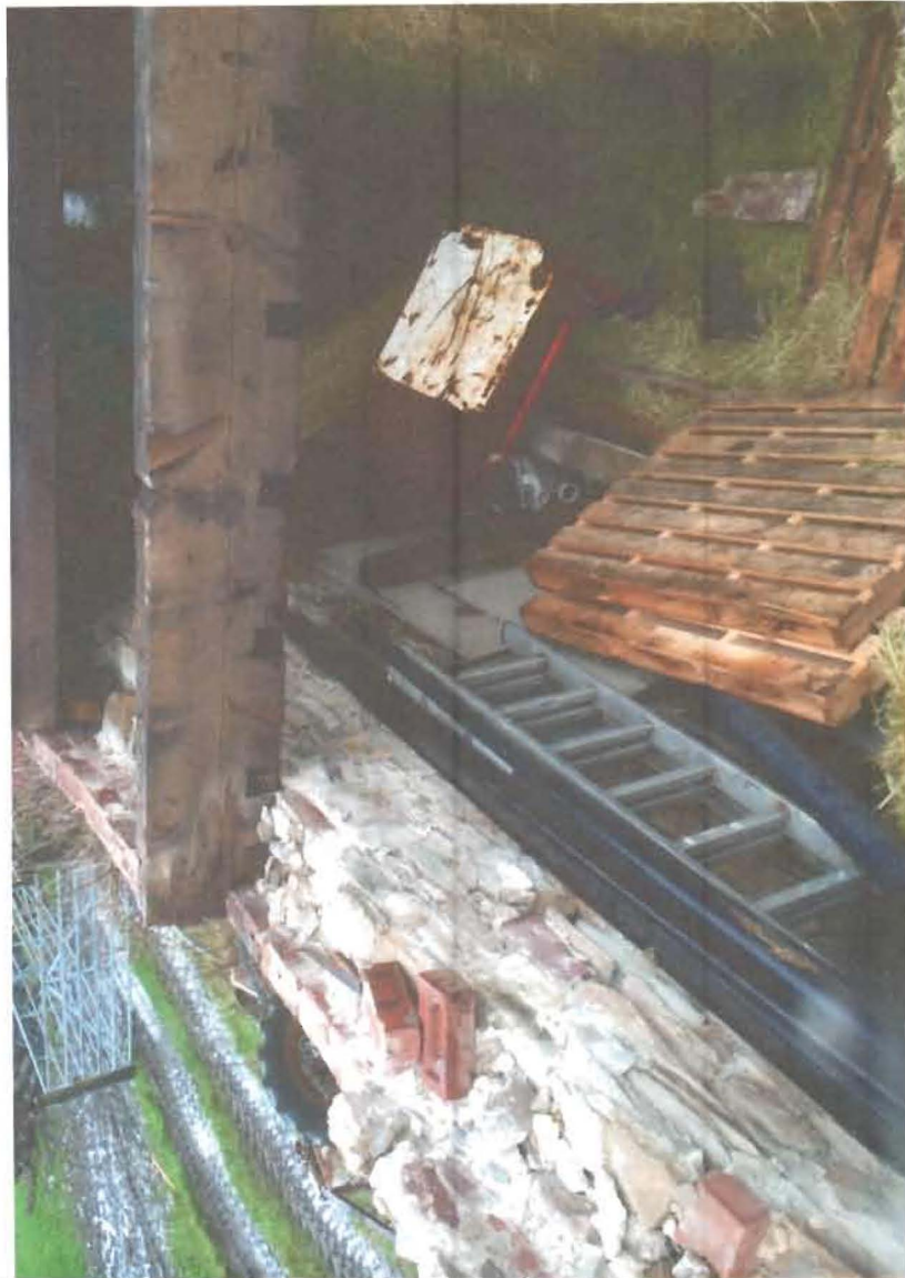
STORM DAMAGED BUILDING.
