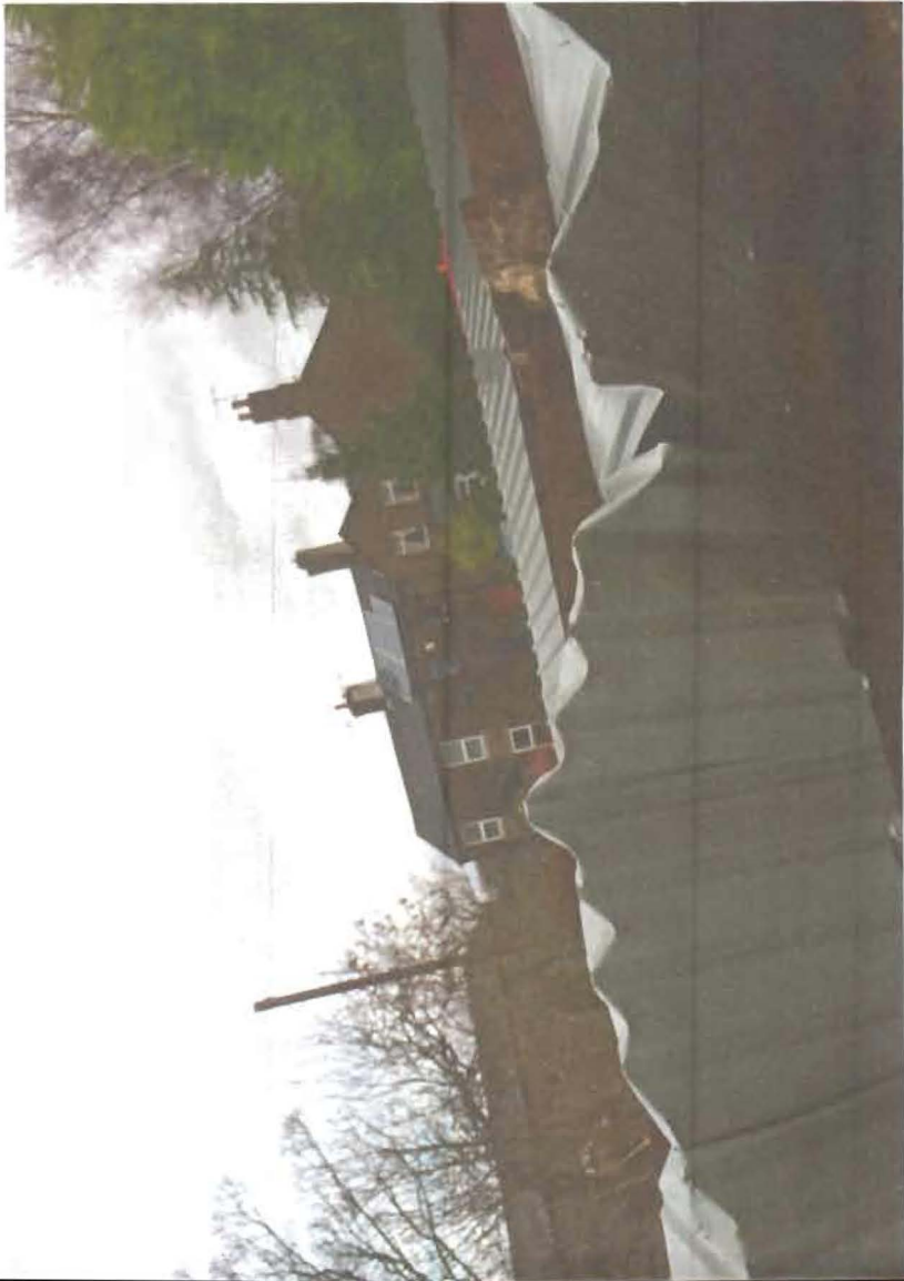
STORM DAMAGED BUILDING.
