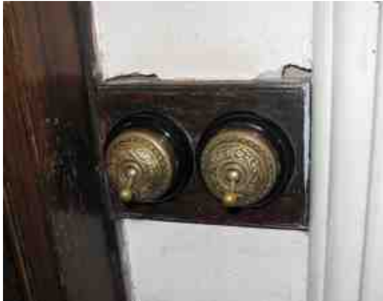
Fig. 41. Original light switch from when the house was converted to electricity and are still in used today.
