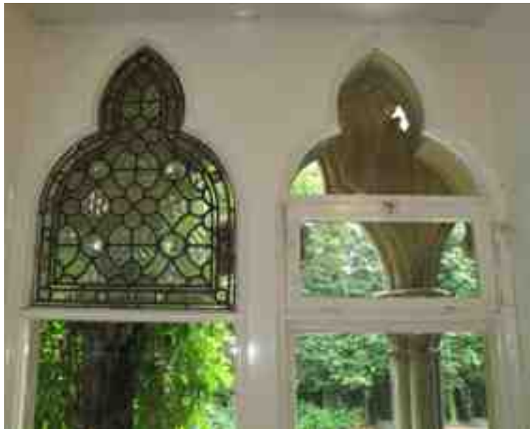
Fig. 40. Windows over looking the verandah from the admin office. Note the right hand window has been altered.
