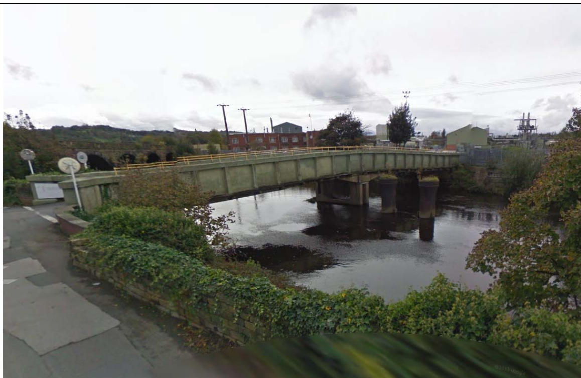
Figure 5.5: Road Bridge downstream of Railway Bridge
