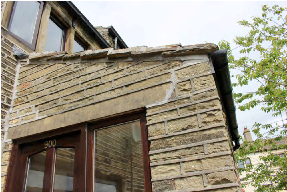
Figure 1.2 – Front Elevation Photograph illustrates cracks, poor quality structure
