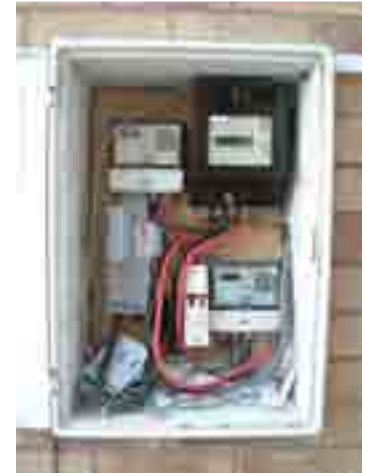
Figure 5. Typical meter box with import and export meters
